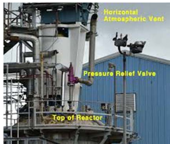
Figure 1. Reactor with a pressure relief system (U.S. Chemical Safety Board, 2018)
