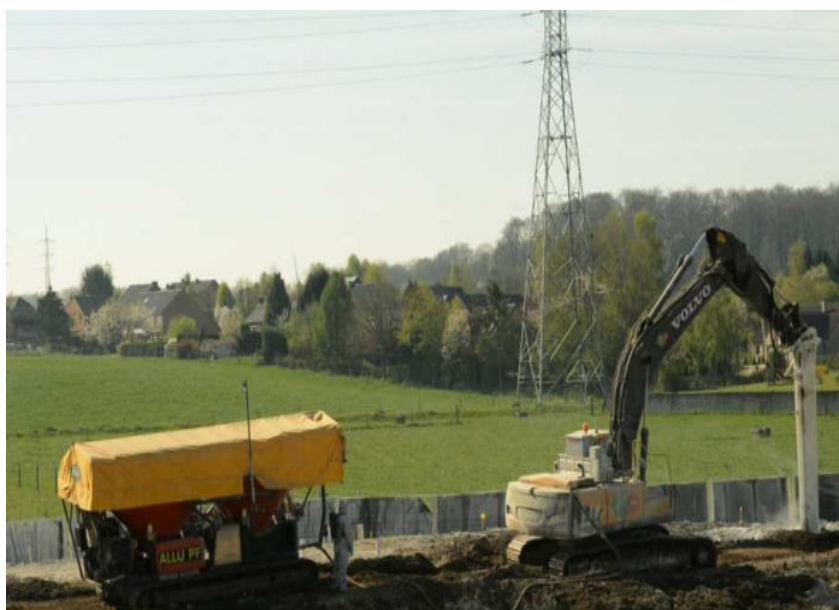
Fig. 4. Equipment used to neutralize the acid tar. On the left, the mobile feeder. On the right, the excavator equipped with the mixer.
