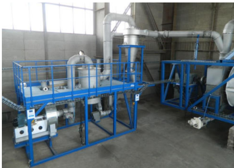
Fig. 5. Off-gas pretreatment module of continuous thermal desorption pilot unit.
